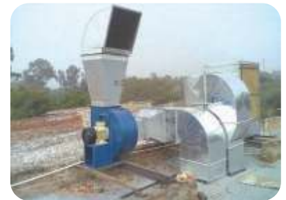
FRESH AIR & EXHAUST DUCTING
